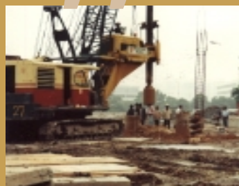
Earthworks and bored piling works to development of new ITE at Bukit Batok
