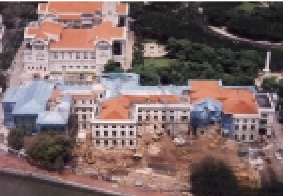
Conversion of Empress Place Building to Second Wing of the Asian Civilisations Museum
